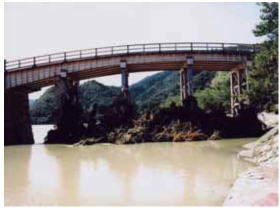
Photo 8: Drift that blocked the water flow under the fifth span
